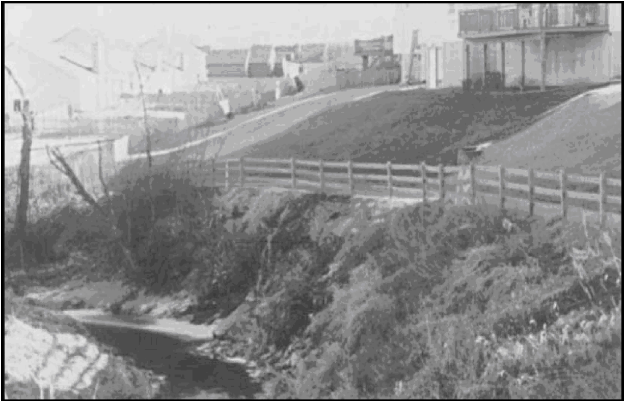
Figure 6.6: Homes too Close to Streambank Source: K. Grimes, SWCD, St. Charles County.
