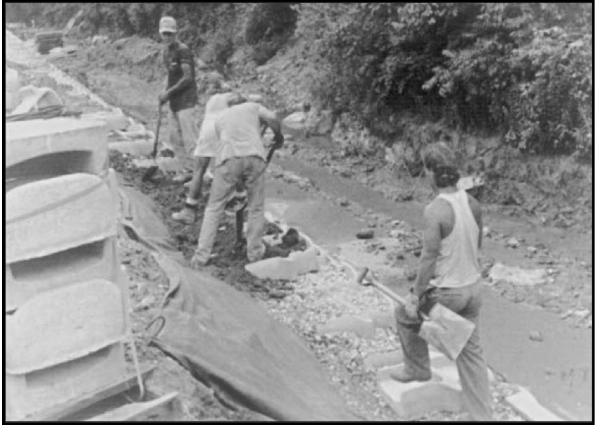
Figure 6.142: Interlocking concrete blocks along Two Mile Creek, St. Louis County. Source: K. Grimes, SWCD, St. Louis County
